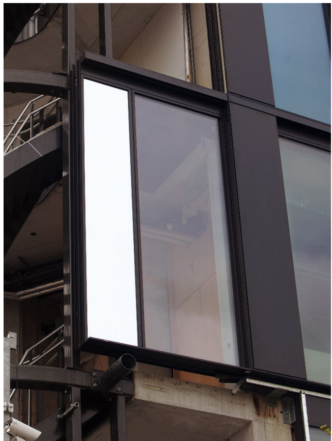
Figure 2: The façade elements with fixed glazing consisting of functional insulating glass are implemented using a special solution based on the HUECK Trigon Unit L standard façade system. The electronically controlled panels were mounted afterwards. (Source: HUECK)
